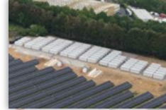
COPWOOD VFB ENERGY HUB 20.7 MWh VS3 / Sussex
