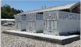
SOBOBA FIRE STATION (CEC) 0.5 MWh VS3 / California
