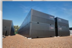
DAIRYLAND (US DOE) 43 MWh Endurium / US Midwest
