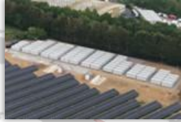
COPWOOD VFB ENERGY HUB 20.7 MWh VS3 / Sussex
