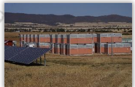
SPENCER ENERGY 8 MWh VS3 / South Australia
