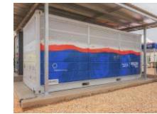
HORIZON POWER 0.3 MWh VS3 / Western Australia
