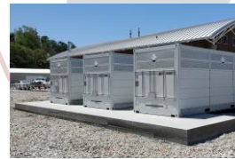
SOBOBA FIRE STATION (CEC) 0.5 MWh VS3 / California
