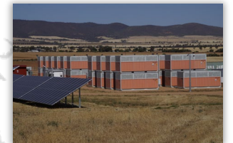
SPENCER ENERGY 8 MWh VS3
