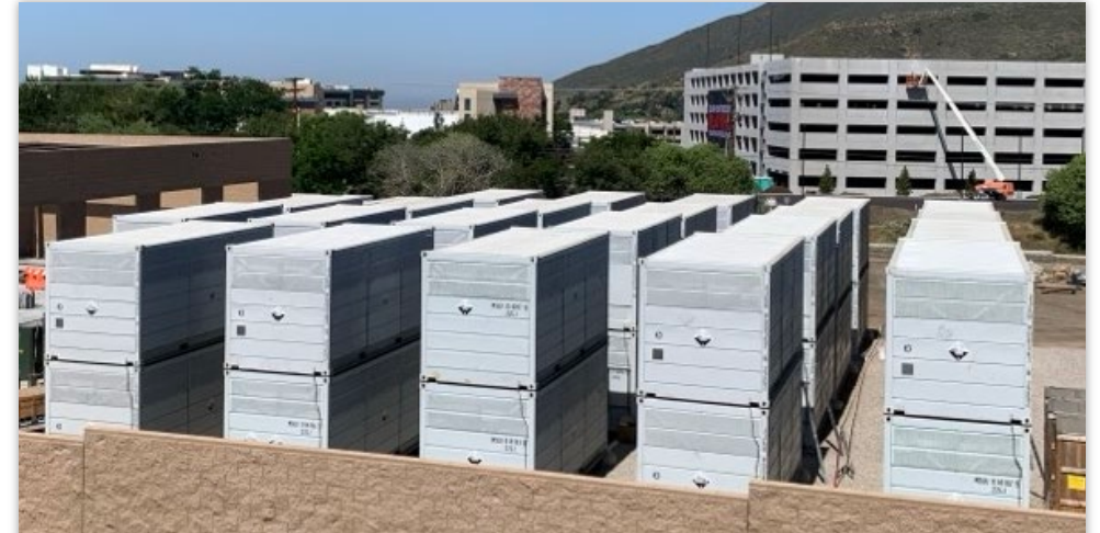
North America's Largest Vanadium Flow Battery / California Microgrid Resilience 10 MWh
