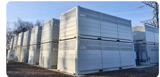
EDF Renewables 5 MWh Oxford, UK
