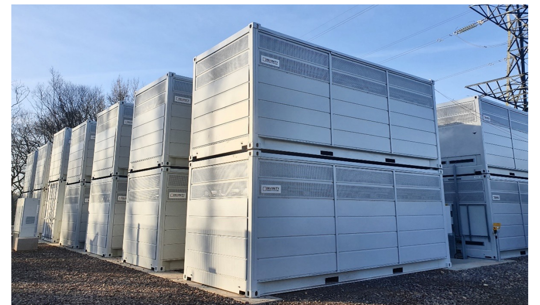
EDF Renewables' 5 MWh Invinity VS3, Oxford UK
