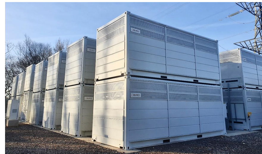
EDF Renewables' 5 MWh Invinity VS3, Oxford UK
