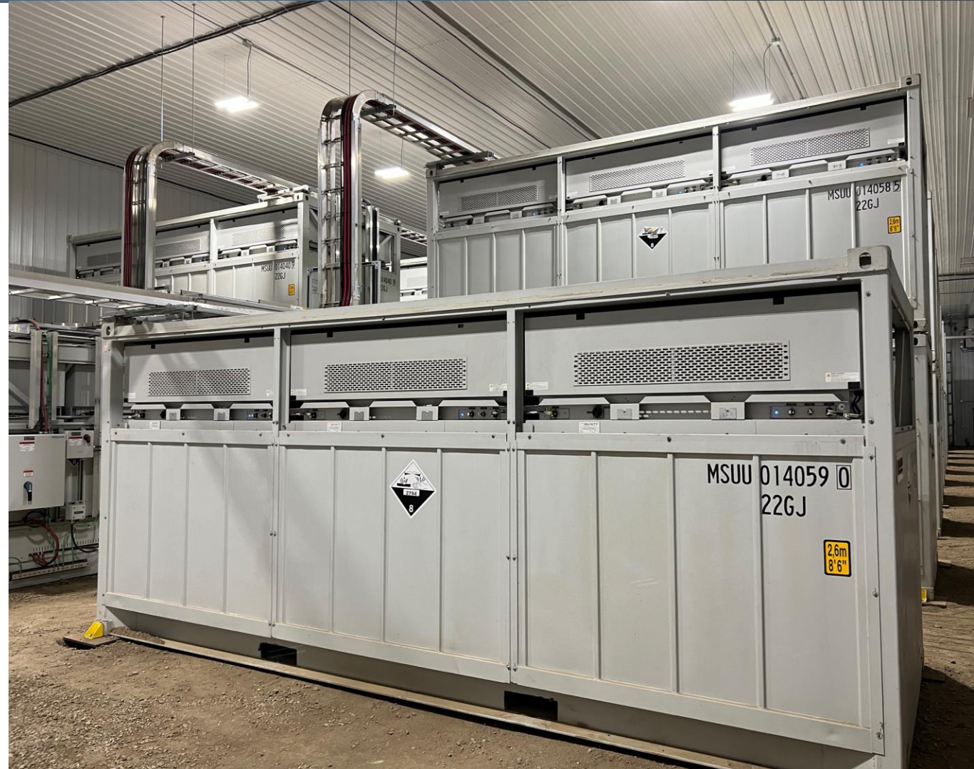
Invinity's Chappice Lake Installation
