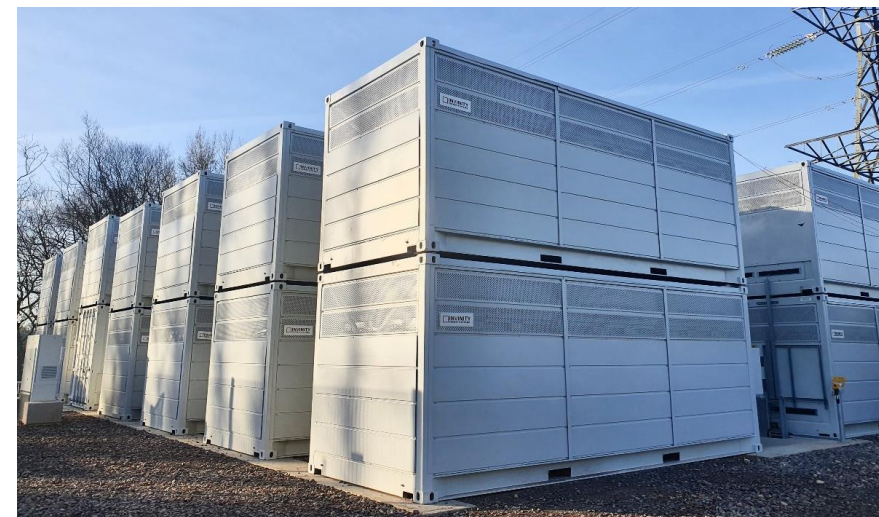
EDF Renewables' 5 MWh Invinity VS3, Oxford UK
