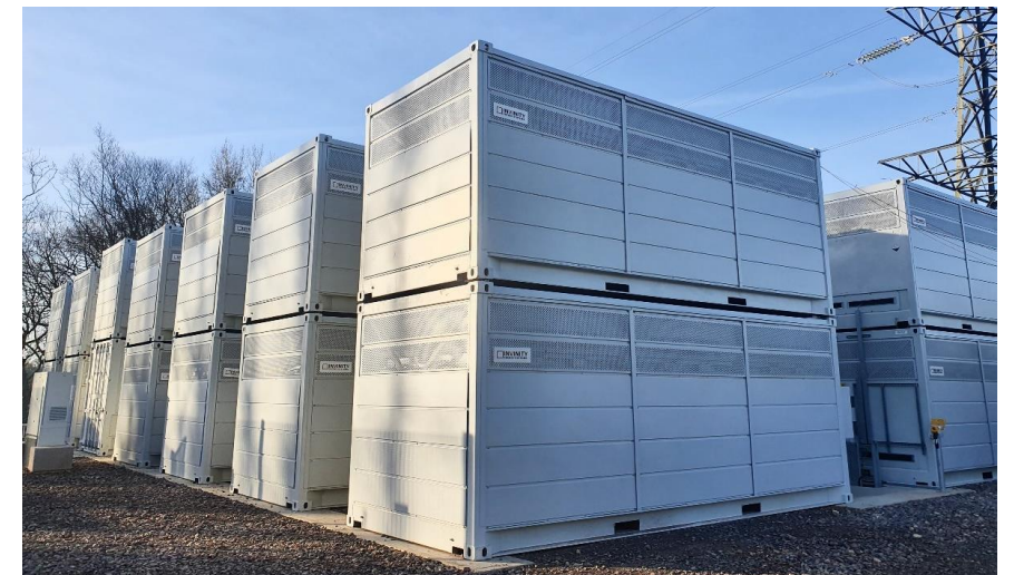
EDF Renewables' 5 MWh Invinity VS3, Oxford UK
